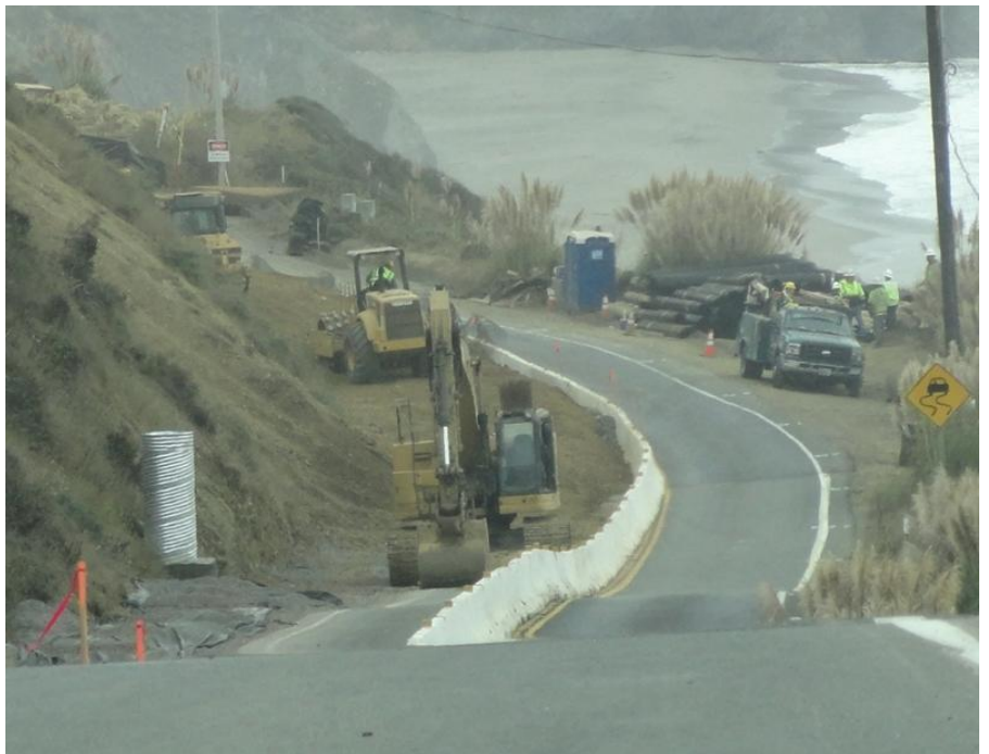
There's a whole lot of diggin' going on at the Westport Slide!
