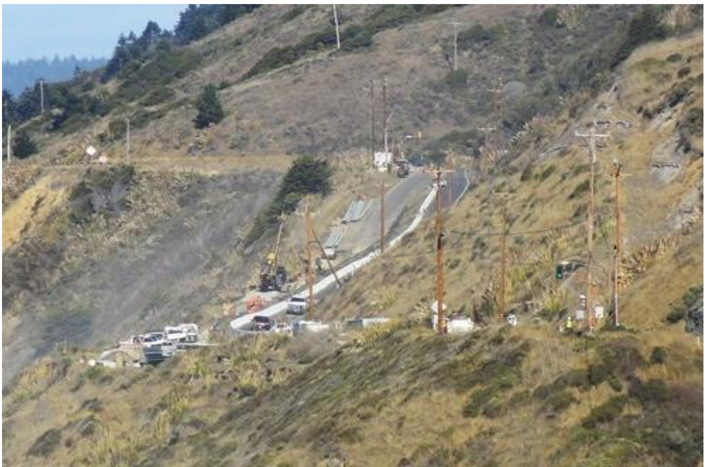
The Westport Slide (and the highway that traverses it) has been slowly moving downhill for generations.
